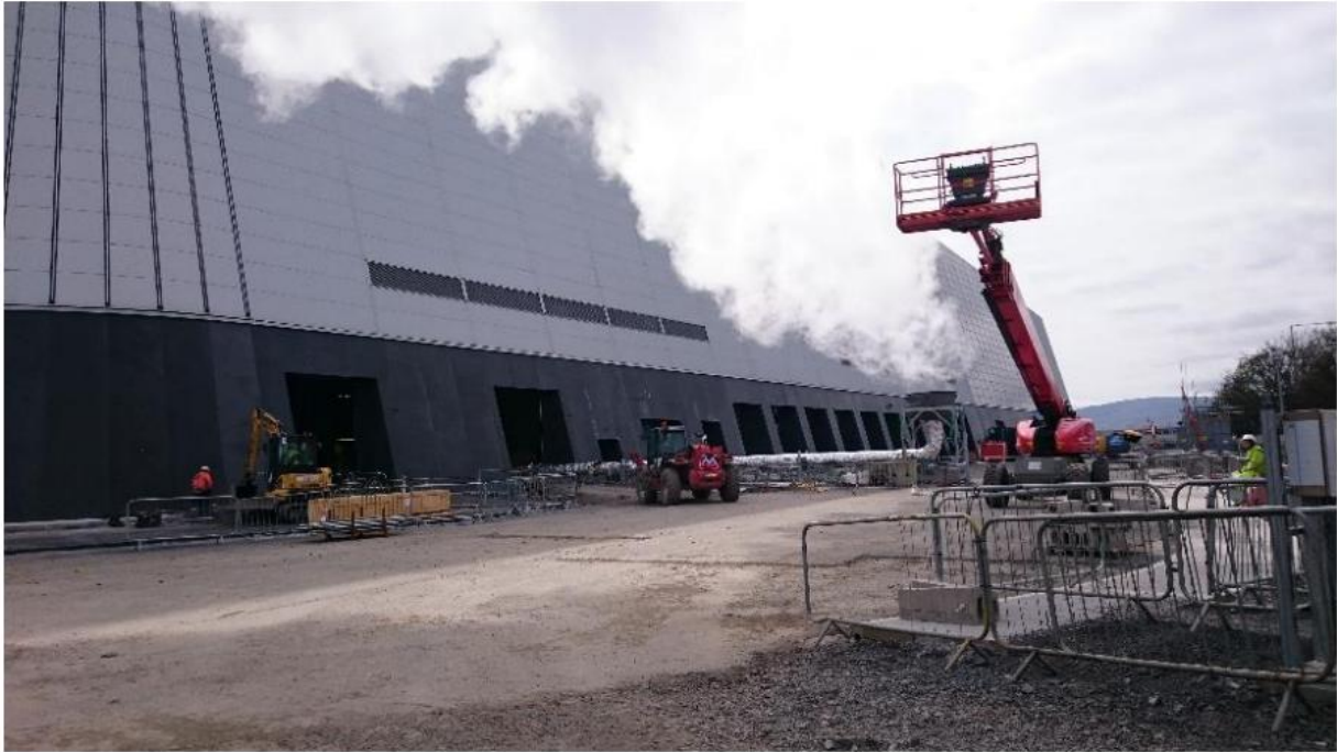
Line 1 - steam blows at the north west of the site (Copyright PML)
