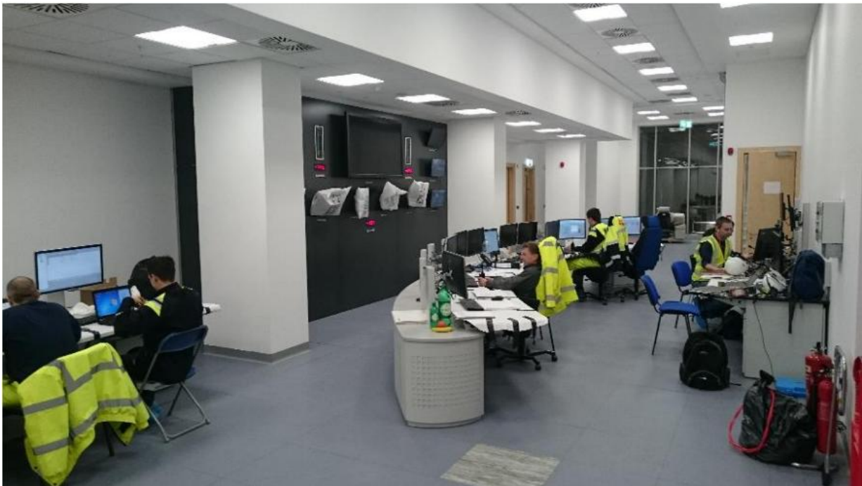
Signal testing ongoing – above photograph shows signal testing ongoing in the control room, located in level 4 of the admin building (Copyright PML).
